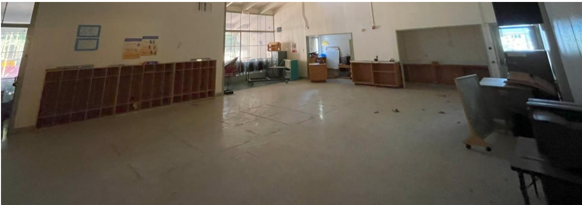
Classroom vinyl flooring is dated and failing.
