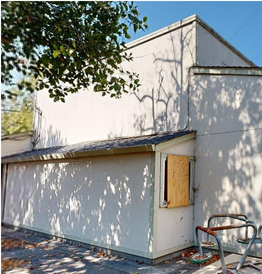
High low-slope built-up roof & damaged window glazing.
