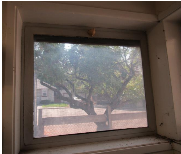
Single-glazed window is not operable. Glazing gasket must be replaced.
