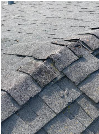
Missing shingles at ridge.
