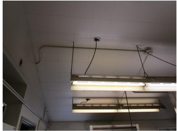
Kitchen sloped glue-on acoustical ceiling tile. Light fixtures are dated.
