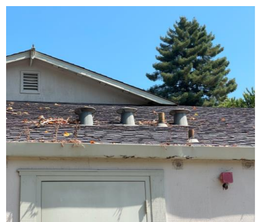
Rusted metal gutter at steep-slope roof.
