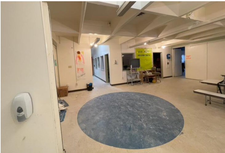
Vinyl flooring in dining area is worn out.
