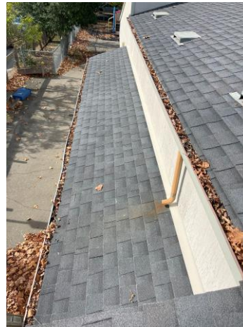
No screen at gutters. Rusted downspout
