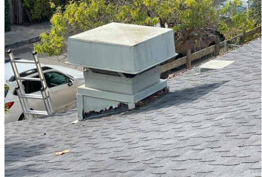
Wood decay at roof curb cladding with insufficient clearance to roofing.
