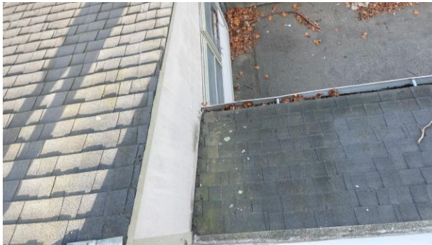
Organic growth on the asphalt shingles. Roofing has reached end of serviceable life.
