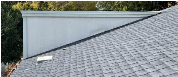
No clearance at base of cladding to roof transition.
