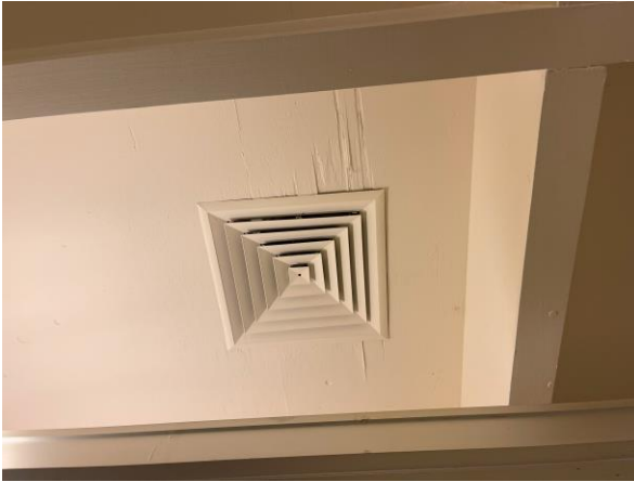
Damaged roof sheathing should be replaced. Roofing above should be patched.
