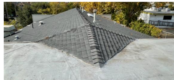
No valley flashing at transition to BUR.
