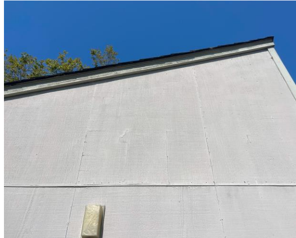
Unsealed joints and cracks at cladding.
