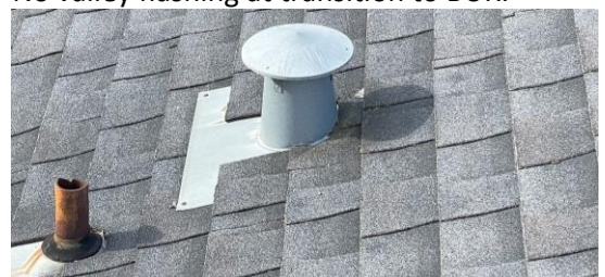
Exposed roofing nails at metal flashing. Rusted pipe penetration.
