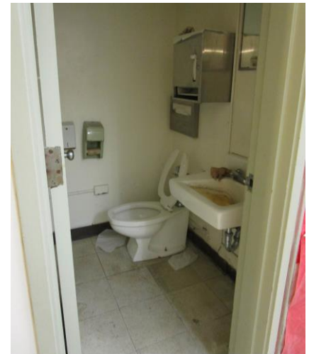
Staff restroom is under-sized. Vinyl flooring is dated and failing.
