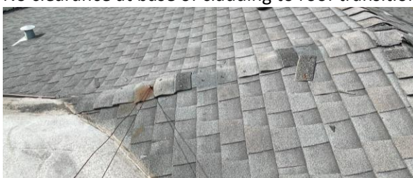
Damaged and missing asphalt shingles at ridge. Exposed roofing nails.
