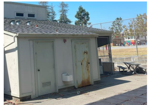
Toy storage door is rusted. Drinking fountain is non code-compliant.
